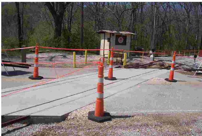
Work still remains to be done on the new crossing but should be ready soon.
