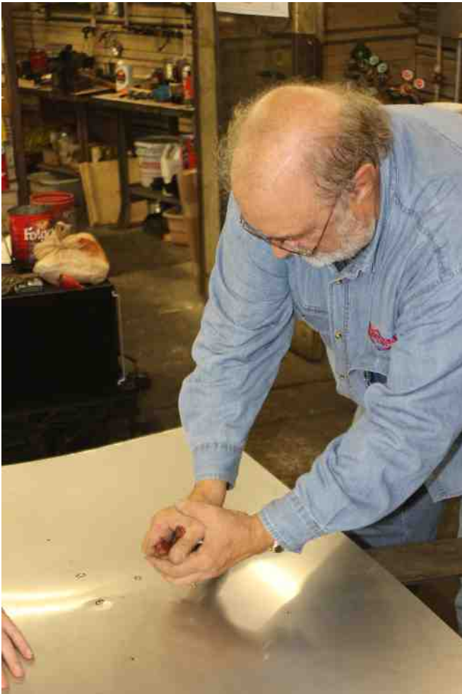
Bob H begins cutting the steel for the fittings on top of the boiler
